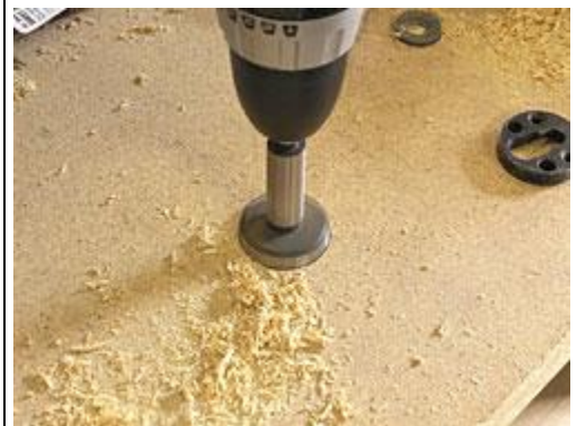
Drilling the 1 1/2" hole (5/16" deep) with a forstner bit for the surface clamp anchor...
